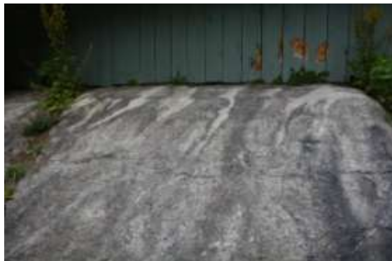
Figure 3a. Frontal view of the runnels under the Visitor Centre.
