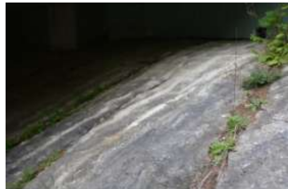
Figure 3b. Oblique view of the same runnels
